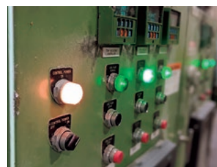
Operation panel of the temperature control system before renewal
