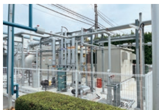
Cogeneration system (Shiga Factory No. 2)
