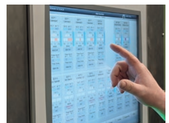
Operation panel of the temperature control system after renewal
