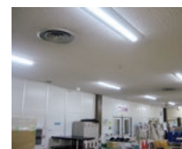
LED lighting bulbs
